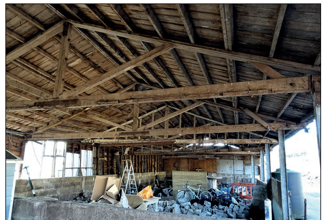
Plate 5 Roof section of Plot 6 showing the timber roof section of a former WW 2 billet, looking west (Image: G.H. Nash).
