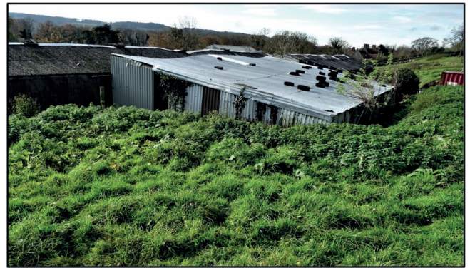
Plate 7 The rear section Plot 5 and the cut into the hillside made for its construction, looking west (Image: G.H. Nash).
