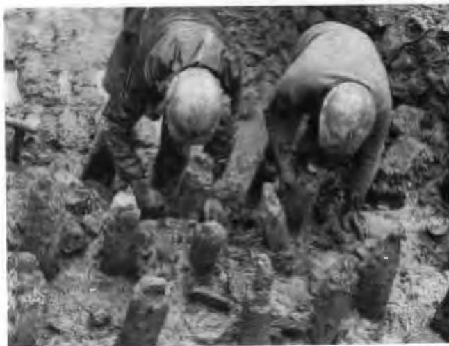
Fig. 9. Wooden piles driven into the soil beneath a wall line to consolidate it prior to building.
