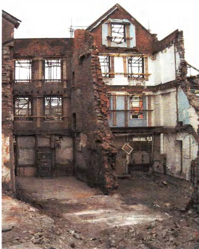
Plate 4 View of Nos. 24 and 26 during demolition showing party wall with 17th-century stonework at ground floor level, looking north.
