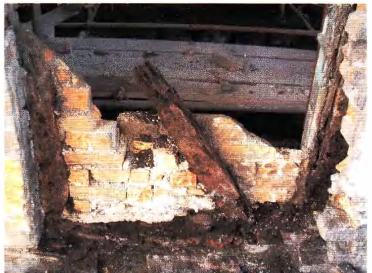
Plate 3 Base-plate (timber 17) supporting post (timber 18) and down brace (timber 10) in bottom north of the eastern boundary wall No. 22.
