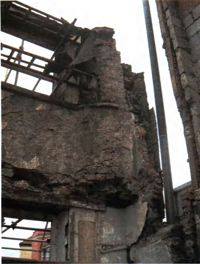
Plate 5 North-eastern corner of No. 30 West Street showing blocked chimney flue at first floor level.
