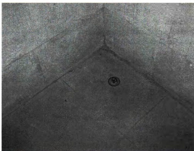
Plate 3 Detail of the plug and drain at the Cold Bath at the Georgian House, Clifton, Bristol.
