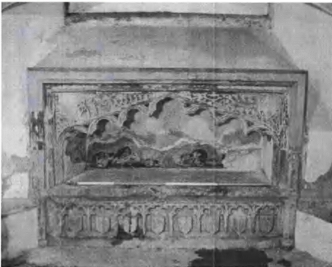
Plate 6 Bay 1 (south) and Chest Tomb G, before conservation, looking south
